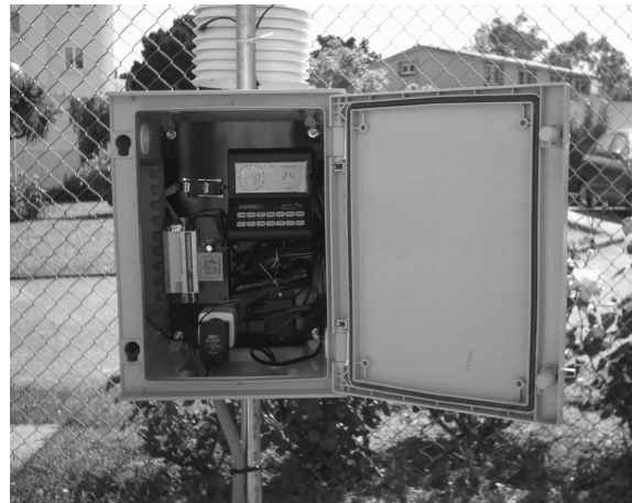
Figure 3: WS data acquisition and communications system assembled in the protection box.
