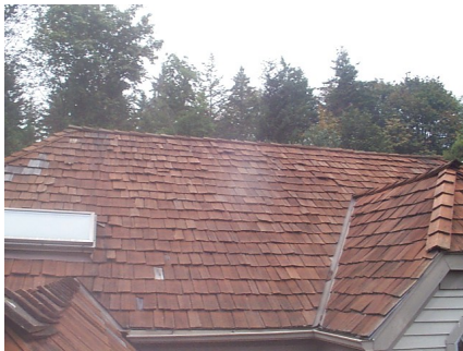
Figure 5: Example of an original image where the roof is a textured surface.
