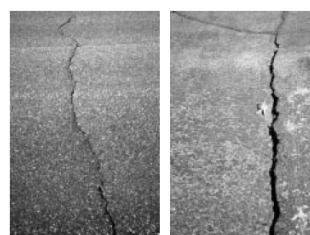
Figure 1: Example of crack on asphalt surface images (transportation information center, 2002).
