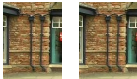
(a) A large structural misalignment. (b) After the segment shift.
