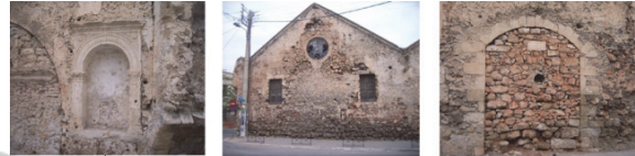
Figure 2: Damaged areas of Neoria in need of restoration.
