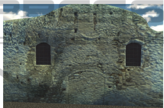
Figure 14: Currently, the door opening is blocked.
