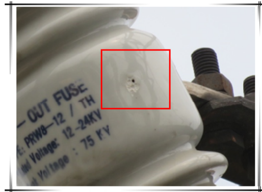
Figure 5: Practice effect of power equipment intelligent detector 1
