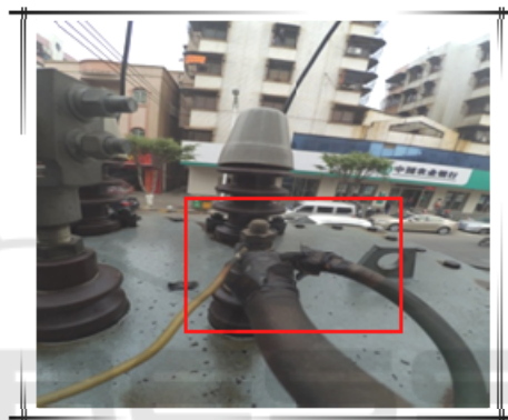
Figure 6: Practice effect of power equipment intelligent detector 2
