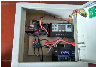
Figure 2: Transmitter box landslide detection.
