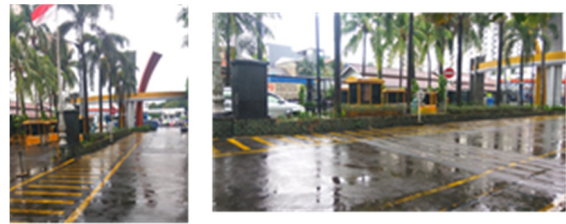
Figure.3. The existing condition of the sidewalk is not free from the vehicle - Before (Segment 1).
