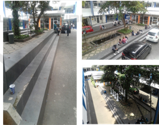
Figure 8: The existing condition of the courtyard sidewalk has not been accessible to the disabled. Before (Segment 2).
