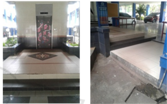
Figure 4: The existing condition of the lobby lift has not been accessible to the disabled. Before (Segment 3).
