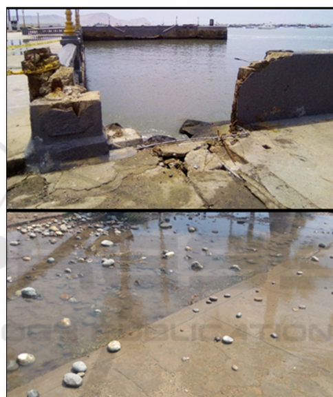
Figure 4: Collapse of the walls of Plaza Grau and stones washed away by the waves. Source: The photograph was taken by the authors in January 24, 2021.
