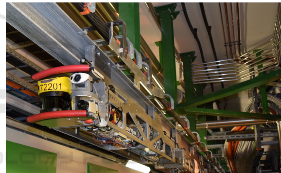
Figure 2: Train Inspection Monorail (TIM).
